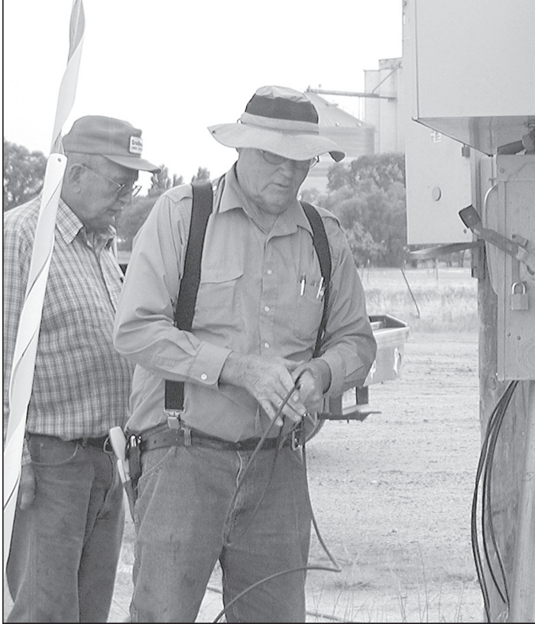
RUNNING ELECTRICAL lines from the boxes to the game booths was at the top of the list for Sam Miller and Kenneth Knorr. The Amusement Authority members have been working, some since the first of the year, repairing rides for the fair. The Amusement Authority will have the carnival open on Aug. 3.
