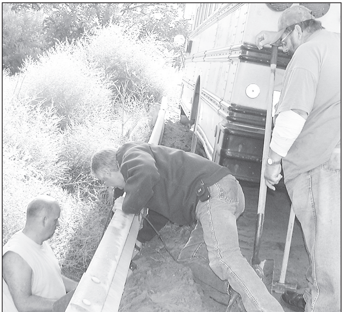
CLOSE CALL — Someone almost had a 20-foot drop Saturday night when they rounded the corner northwest of St. Francis and about missed the bridge completely. The county road and bridge crew were fixing the damage Monday morning. Pictured, left to right, are Ben Killinsworth, Dave Flemming and Mike Antholz.
