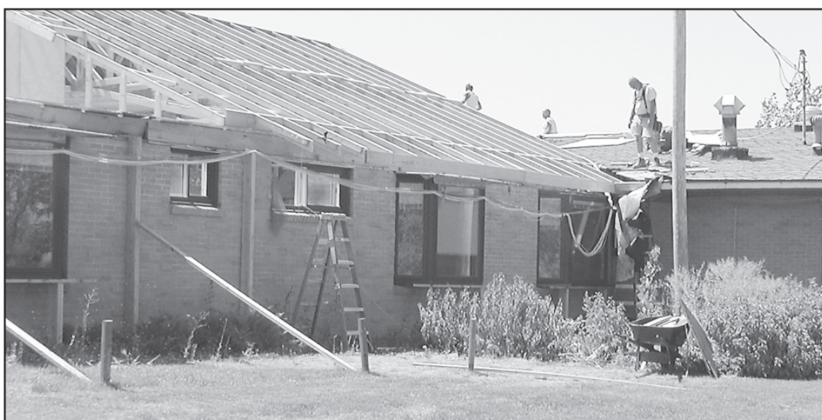
PROGRESS HAS BEEN SLOW but a year after the fire at the Good Samaritan Village, there are many changes seen. On Oct. 19, firemen rushed to the Village to put out the fire; above, workmen started putting on the roof in the spring; workmen on Tuesday were putting the windows in the hallway which is complete enough that Janie Schulz, who works in the kitchen, is able to take the food cart through to the west wing where residents are fed.
