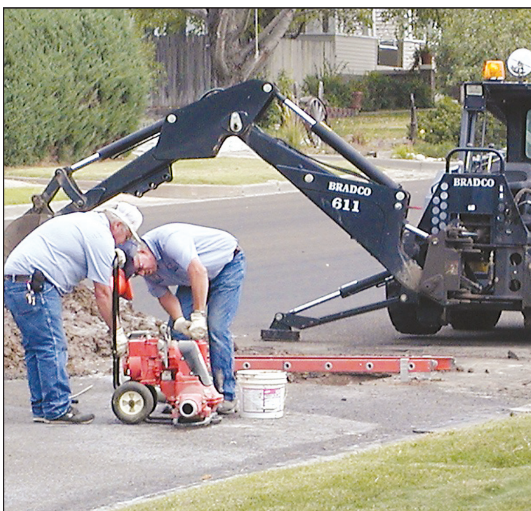
WATER LEAK on East Jackson Street found city workers, Glenn Schliep, left, and Earl Hankins working at the site Tuesday afternoon.
