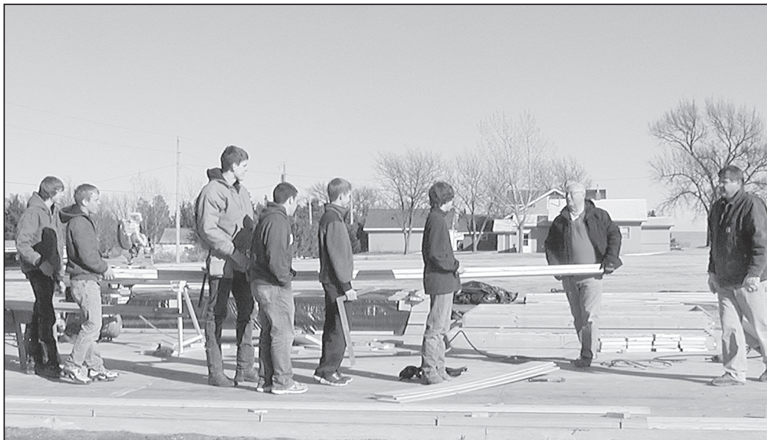
Cheylin students and residents are busy working on the wellness center project being built in Bird City.
