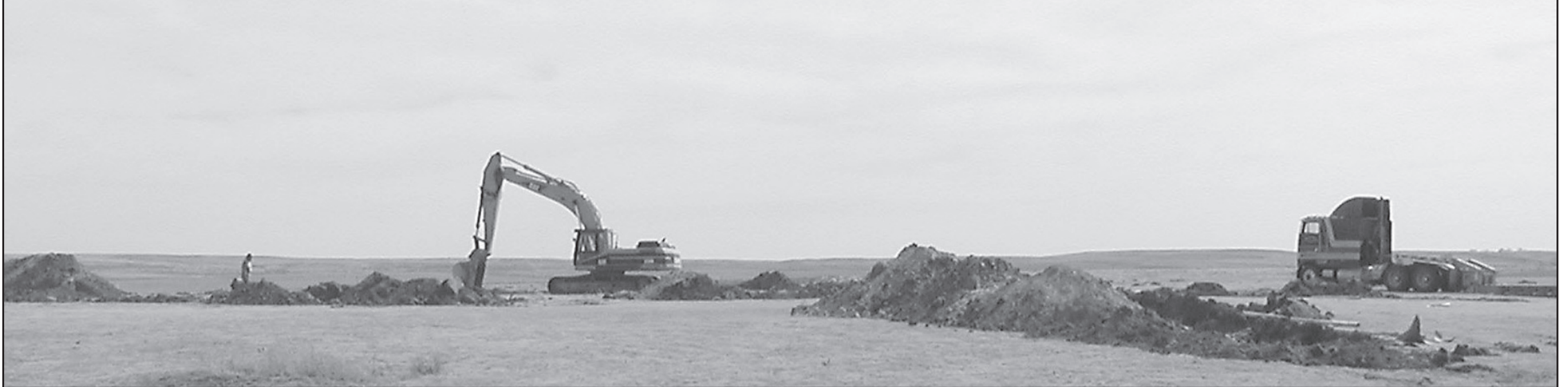
CAHOJ EARTHMOVING crew started the dirt work for the new PrairieLand Electric facility to be built east of St. Francis on U.S. 36.
