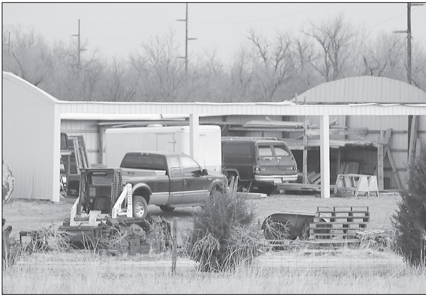
STRONG WINDS clocked between 35 and 45 miles an hour were constant on Sunday. A fire in Yuma County, Colo., burned miles of grassland and sent three firemen to the hospital. Above, the winds took the roof off of a building belonging to Troy Porter on the Angle Road west of St. Francis. Herald staff photo by Tim Burr
