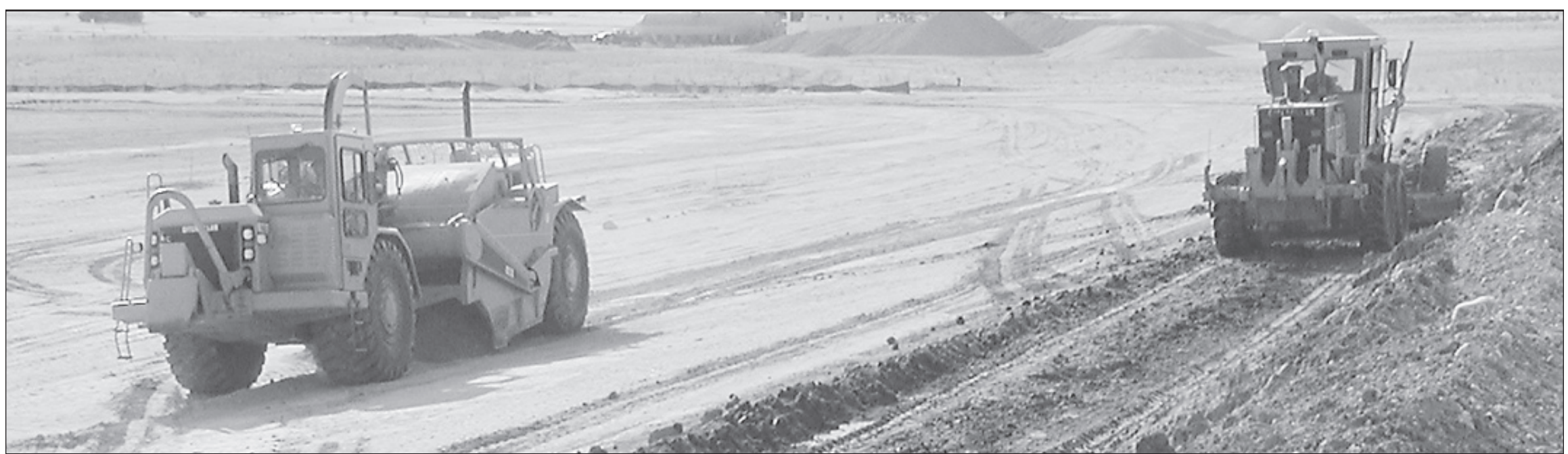
GROUNDWORK HAS RESUMES at the Cheyenne County Airport. The runway will be longer and wider. Construction is expected to be completed by the end of July.
