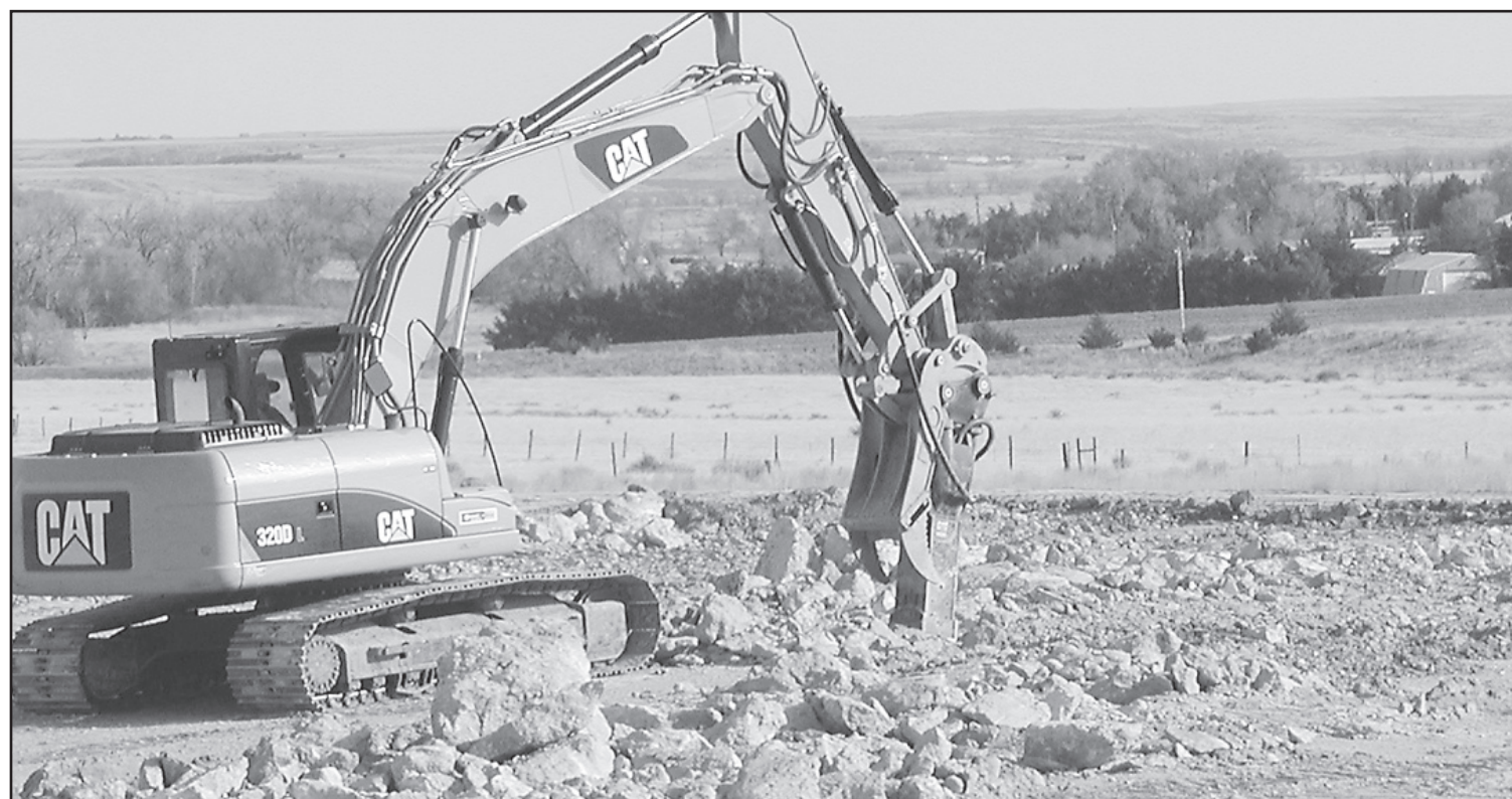
SOLID ROCK was found under a portion of the runway extension. This huge jack hammer was clearing away the rocks and trucks were hauling it off so the dirt work could be done.
