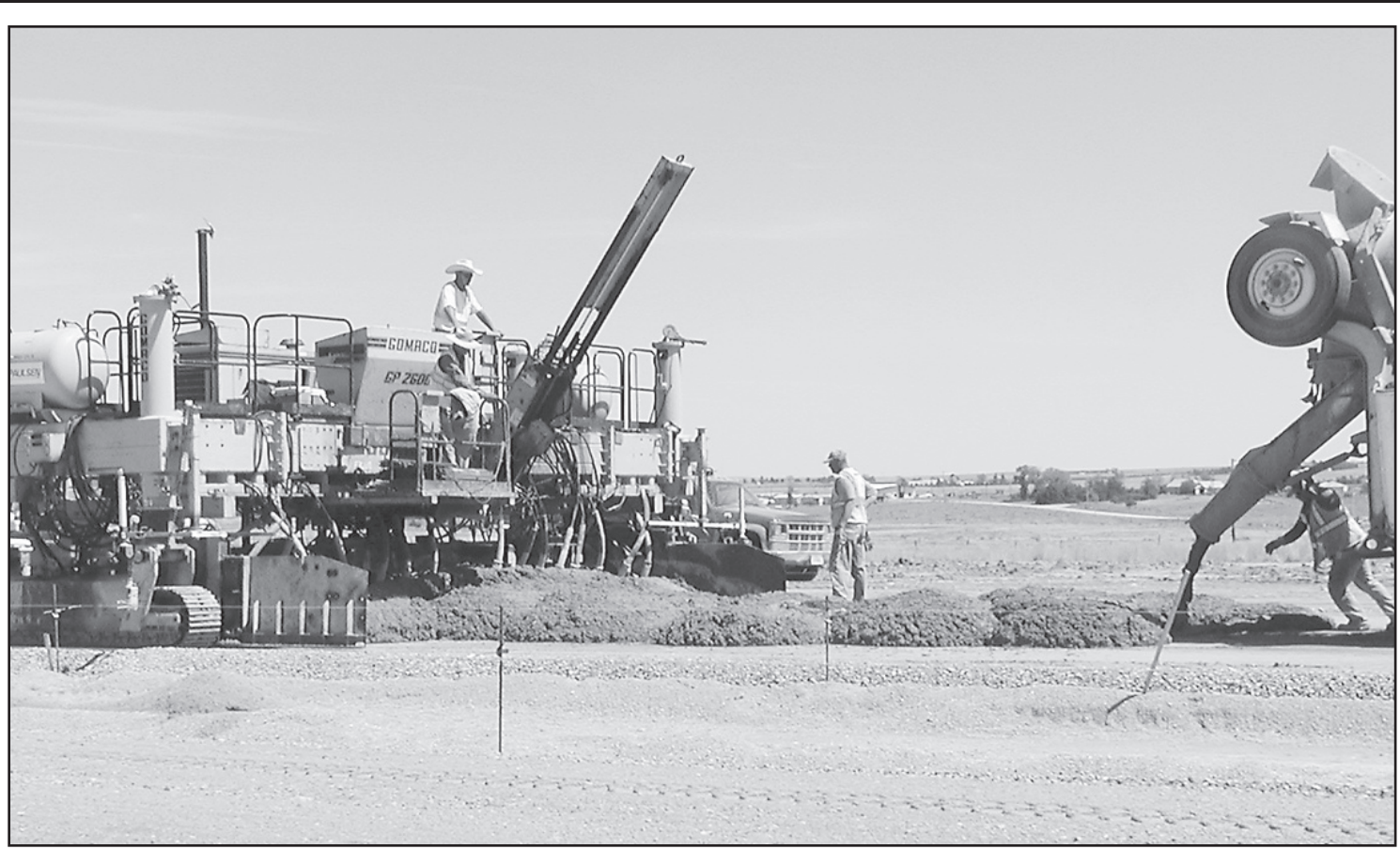
WORK IS MOVING QUICKLY at the Cheyenne County Airport as the workers run the cement for the new runway. The runway will be longer and wider, allowing bigger planes to land safely. Herald staff photo by Tim Burr
