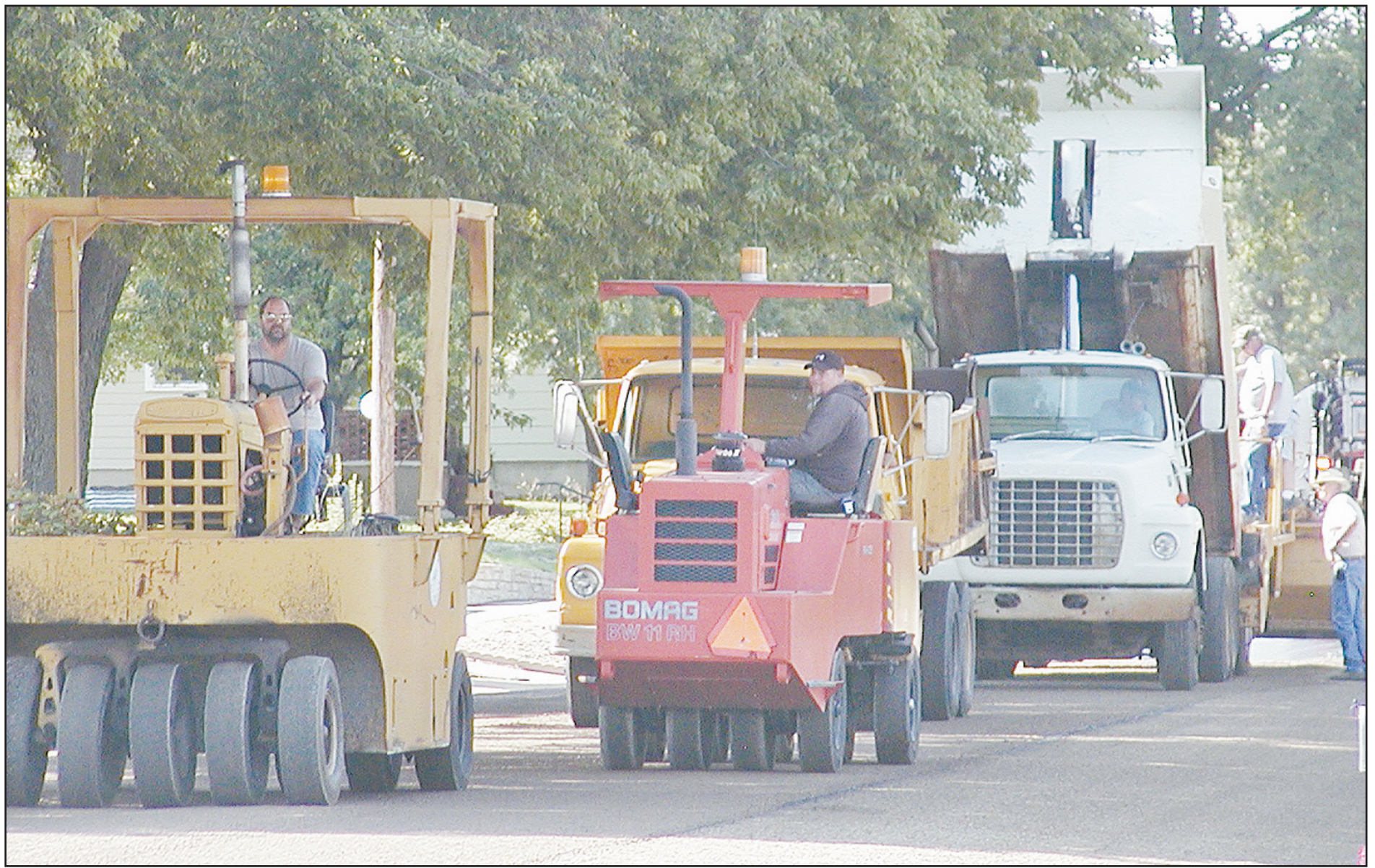
COUNTY AND CITY EMPLOYEES worked together this week to do some road construction on several of St. Francis' streets. The chip seal was applied this week and once it weathers, a fog seal will be applied.
