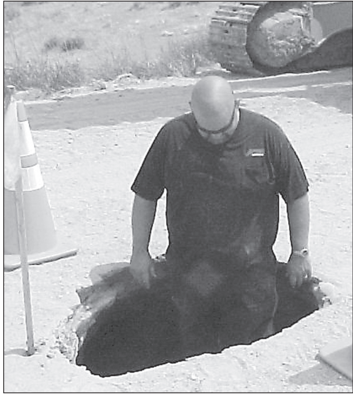
J.W. MILLIKEN, member of the county road and bridge crew, stands in a hole that was found in the road north of St. Francis. Herald photo by Dave Flemming
