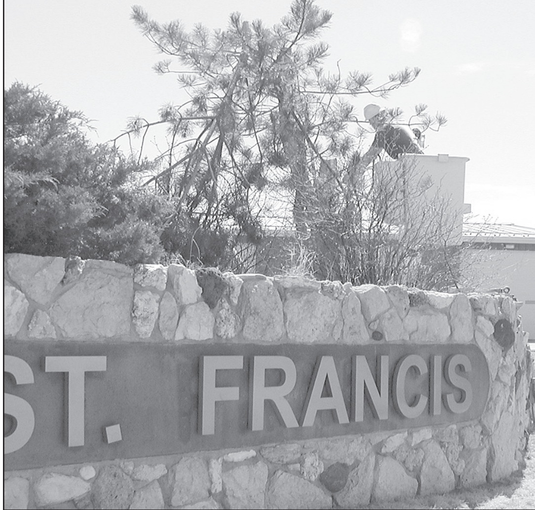
CITY CREW PREPARES berm for the new St. Francis sign. The sign is to be up and lighting the way to Saintry activities by June 15.
