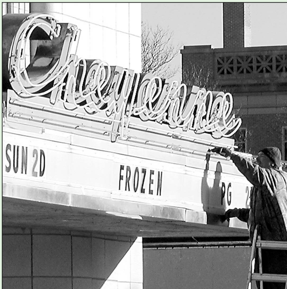
A WORKMAN CAREFULLY removed the old neon gas tubes and then the background of the sign was painted black. People are urged to check out the new lighting on the old sign.
