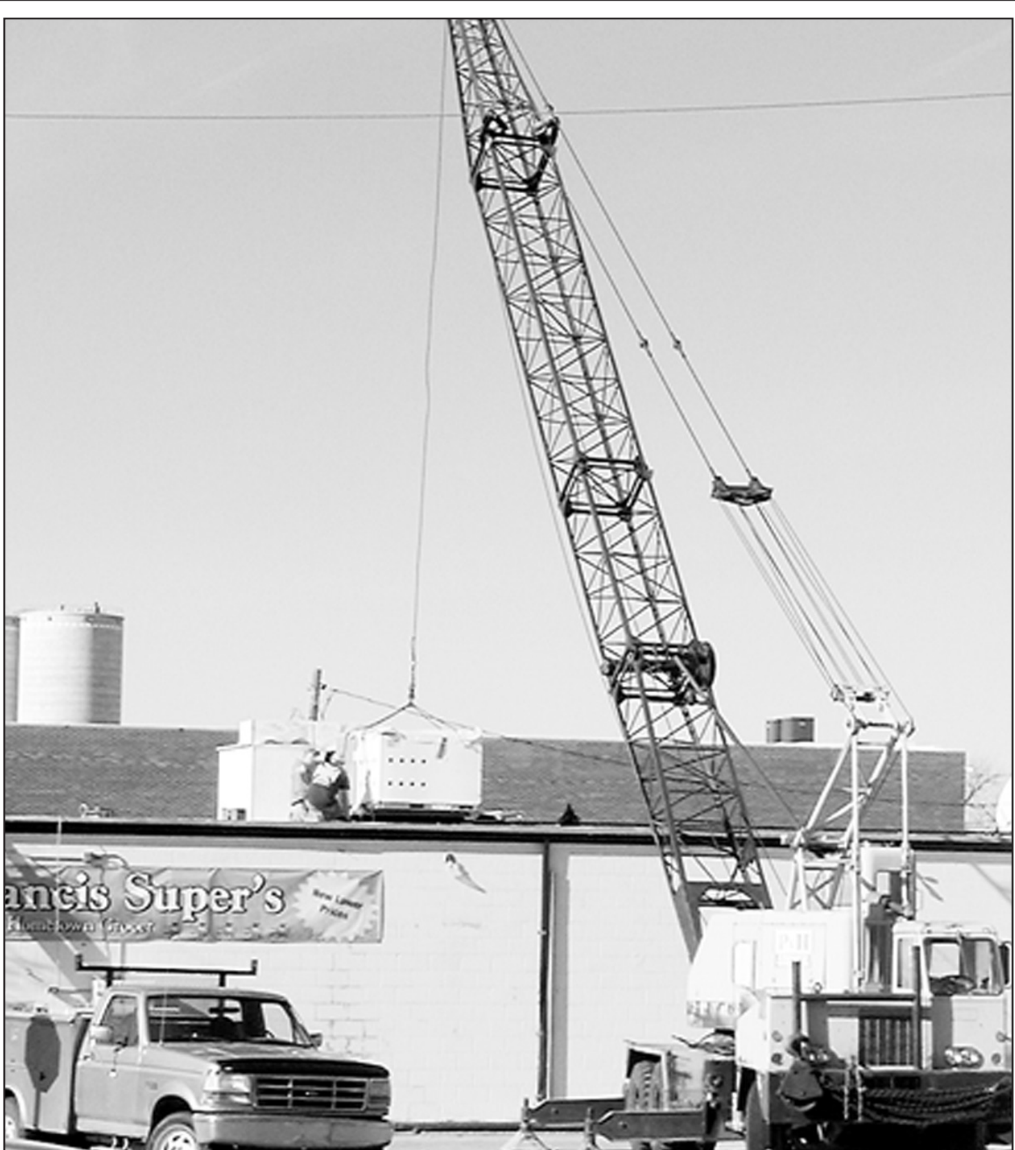
THE COUNTY'S CRANE was evident last week as it lifted the new heating and air conditioning unit to the top of St. Francis Super's and lowered the old one. Getting it set and ready to hook up are Ed Marin and Terrence Lamb with Heartland HVAC, St. Francis.
