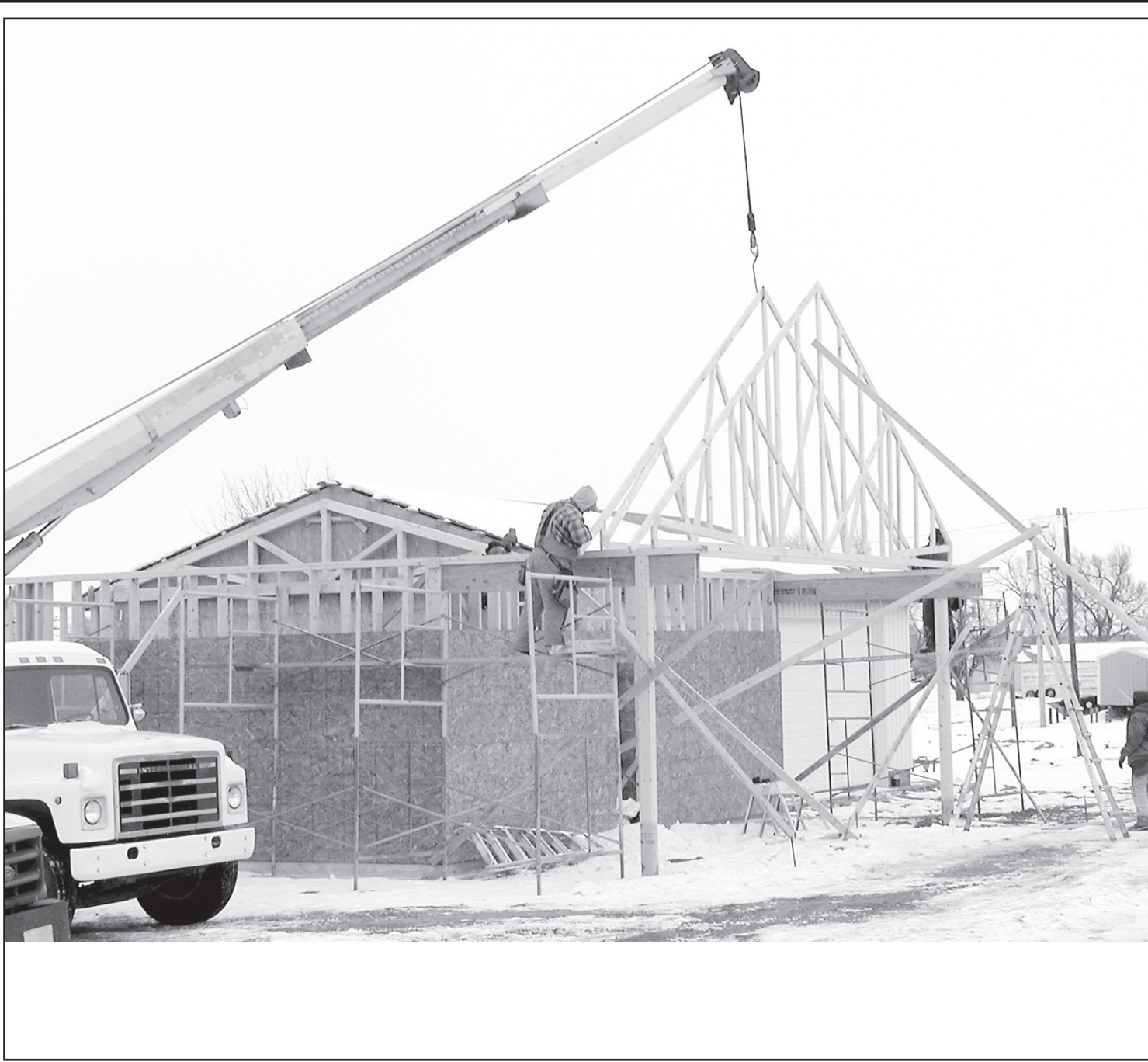
WORKERS CONTINUE at a frantic pace to complete the B&W building on Highway 36.
