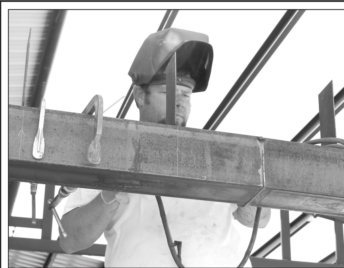
ANDY LIMING and his crew from Wray Colo., are diligently working on the new Wright Building to have it ready for the Thresher Show. Andy was welding the loft framework, and his crew members were working in the heat on the roofing. Mr. Liming said the building should be done in time, the only hangup might be with the electricity.
