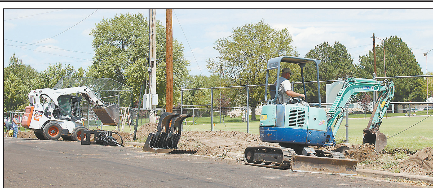
BROCK MCATEE CONSTRUCTION was busy tearing out the sidewalk Monday afternoon to the west of the grade school. A new sidewalk will be in place by the time school starts this year. Herald staff photo by Amanda Miller
