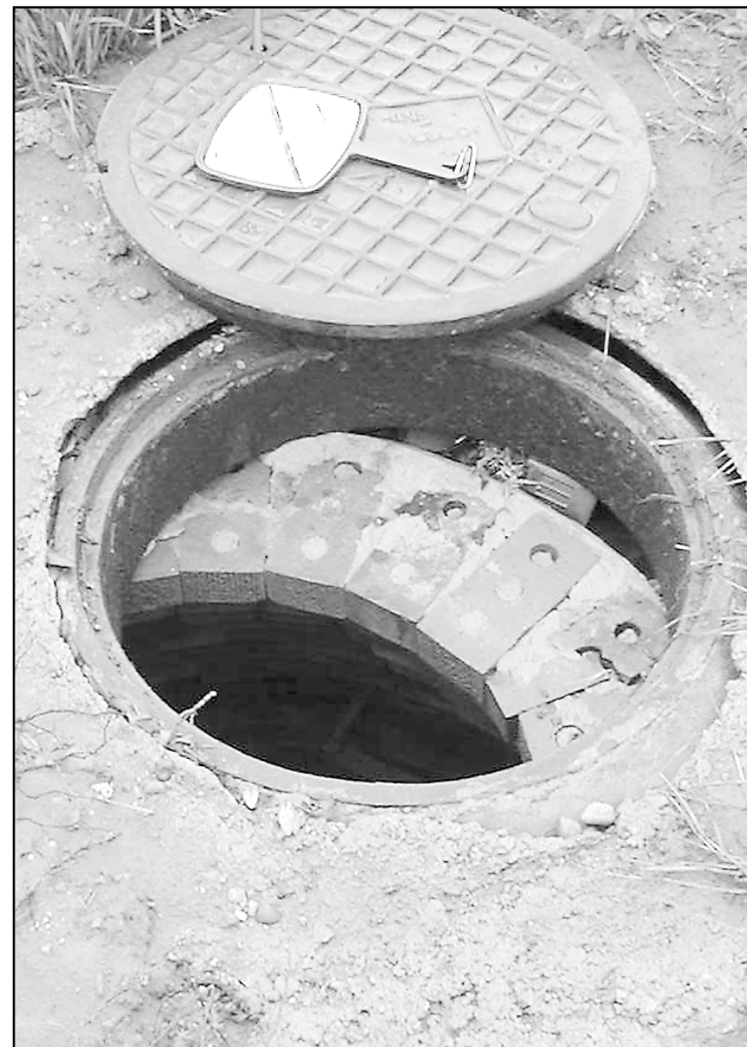
ONE OF 80 MANHOLES that need repaired is pictured above. This manhole is not placed right and water runs through the hole at the top.
