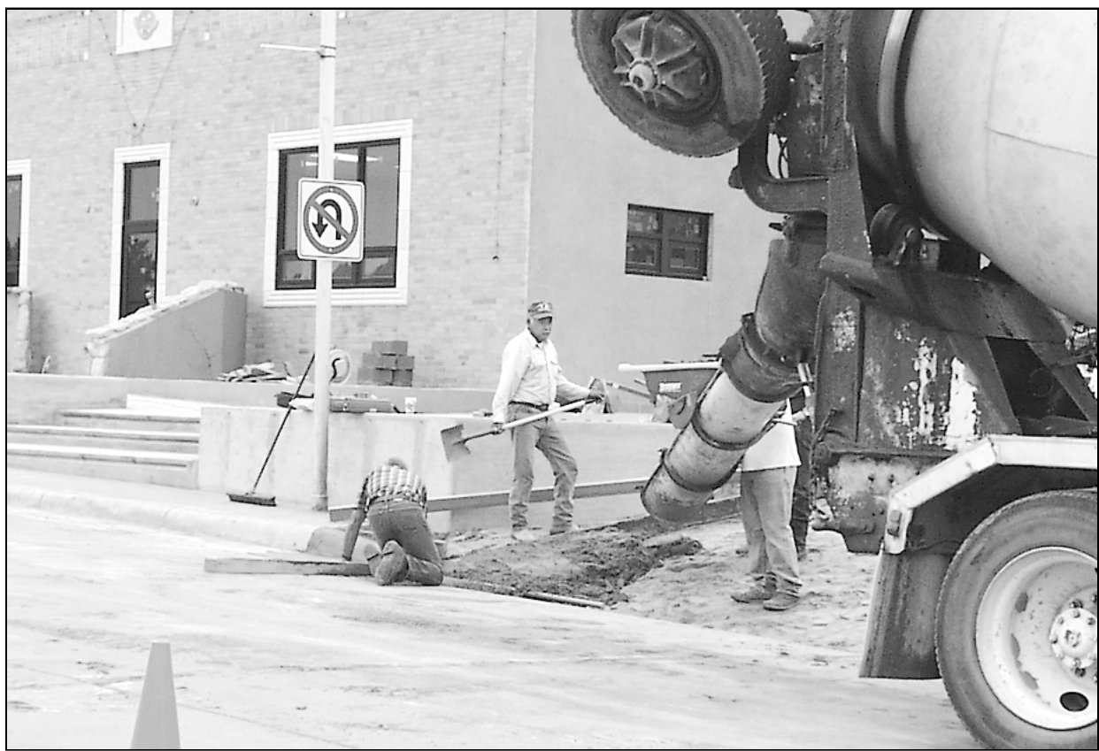
LANDSCAPING IS UNDERWAY at the new city hall building on East Main Street. Troy Porter and his crew will be adding small trees and shrubs to enhance the historical building.
