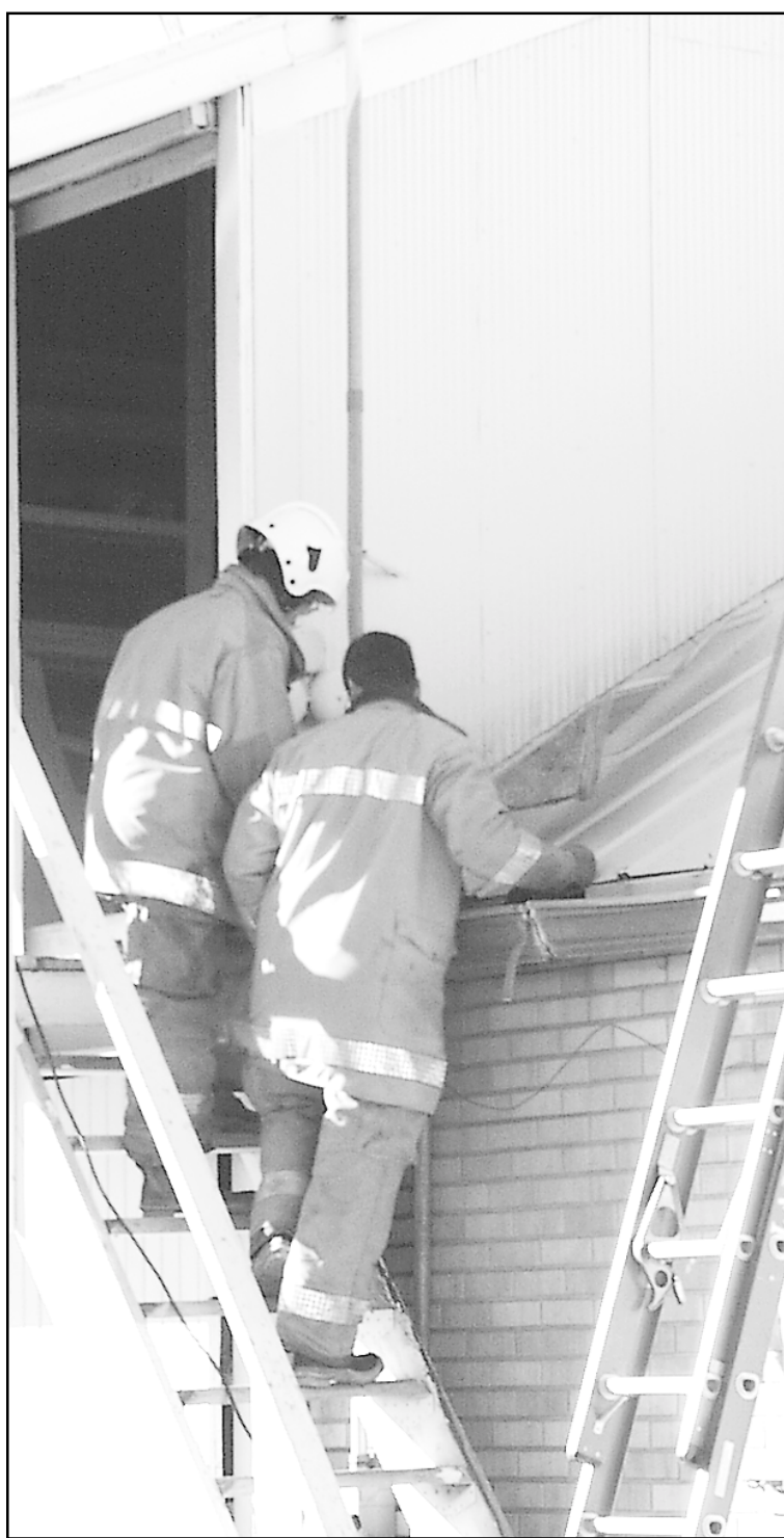
VOLUNTEER FIREMEN Sam Miller and Rob Schiltz investigated the fire that started at Tri-State Lumber on Friday after a piece of gutter was cut with a torch. There was little damage reported. Herald staff photo by Karen Krien
