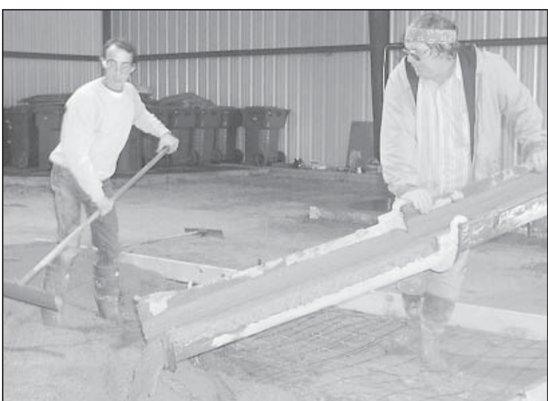
DONATING THEIR TIME — John Amack, right, and his helper Jeff Fryburger are running the cement floor in the city's recycling building and have volunteered their labor.
