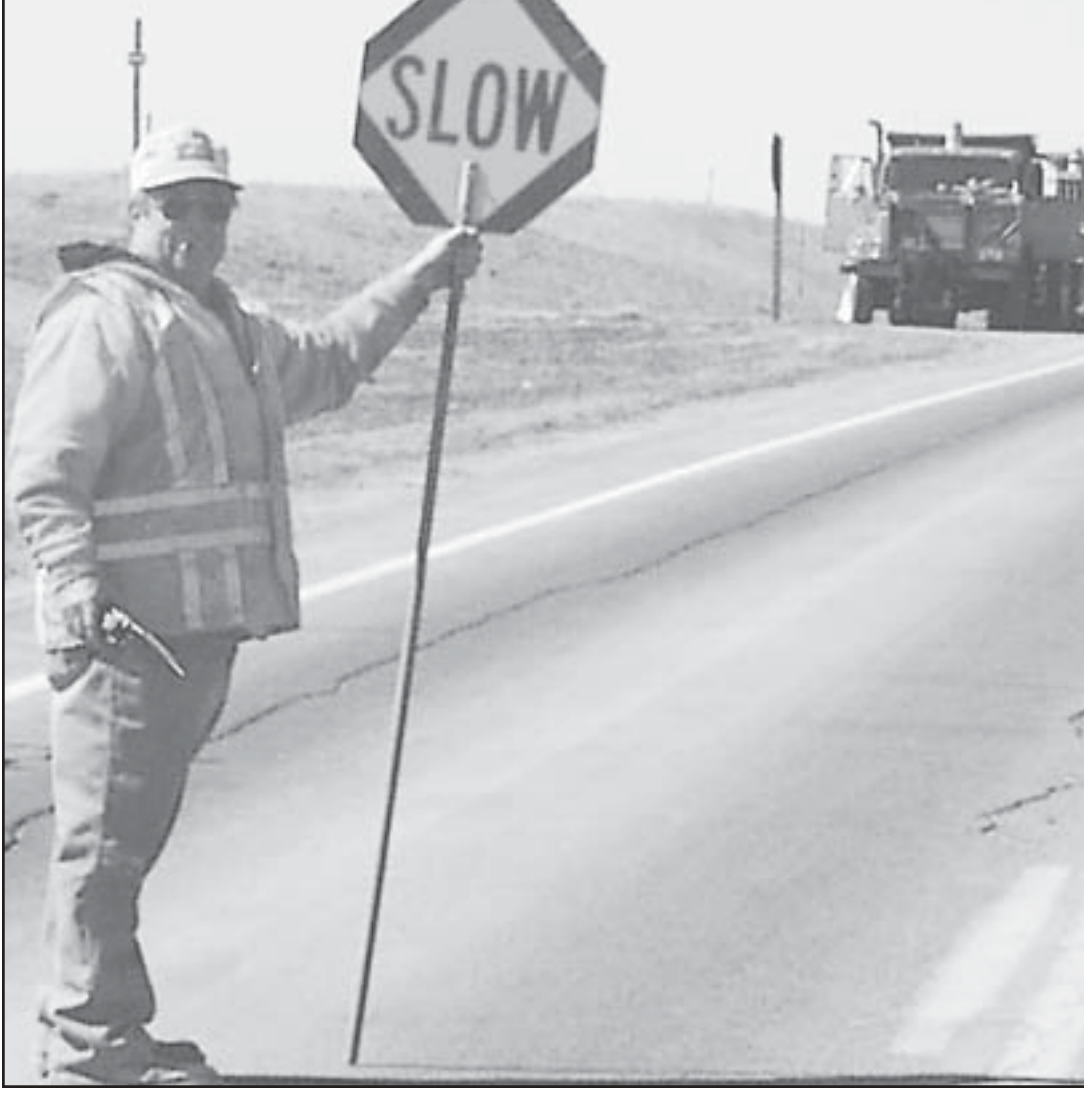
ROAD WORK is going on east of Wheeler on U.S. 36. Larry Zwegardt, state crewman, was stopping traffic Tuesday afternoon. Herald staff photo by Karen Krien
