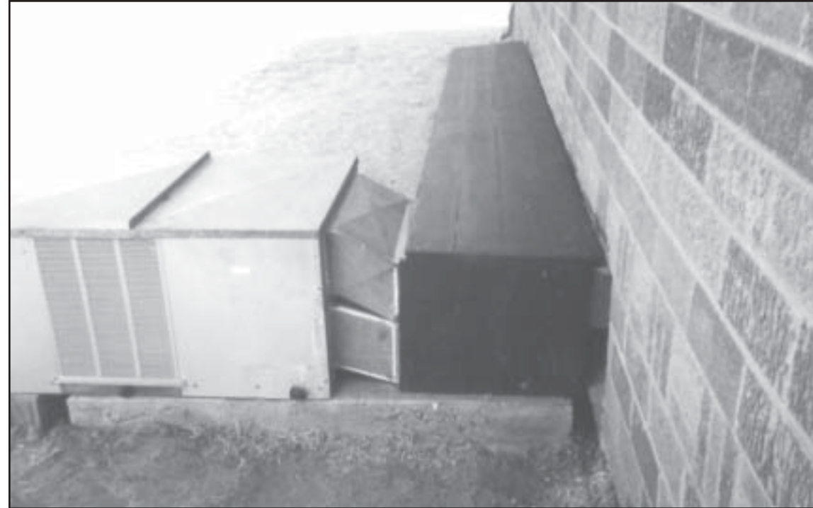
REPLACING THE casing around the heat/air conditioning at the Clough Valley Church was Joel's final project before achieving the rank of Eagle Scout.
