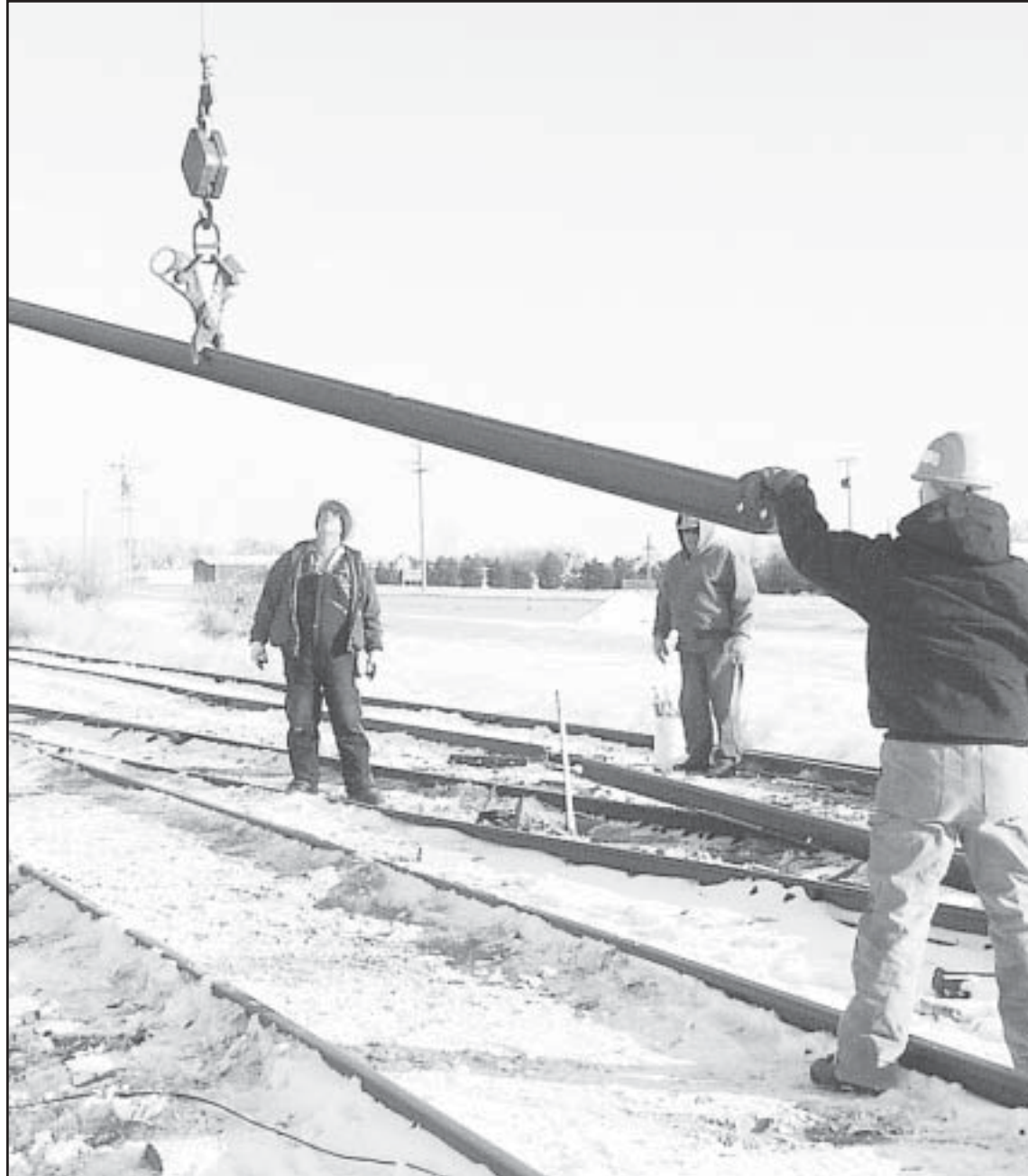
WORKERS FOR THE Nebraska-Kansas-Colorado Rail Road fight the elements to repair damaged tracks from a derailed tank car west of Bird City. Times staff photo by Casey McCormick
