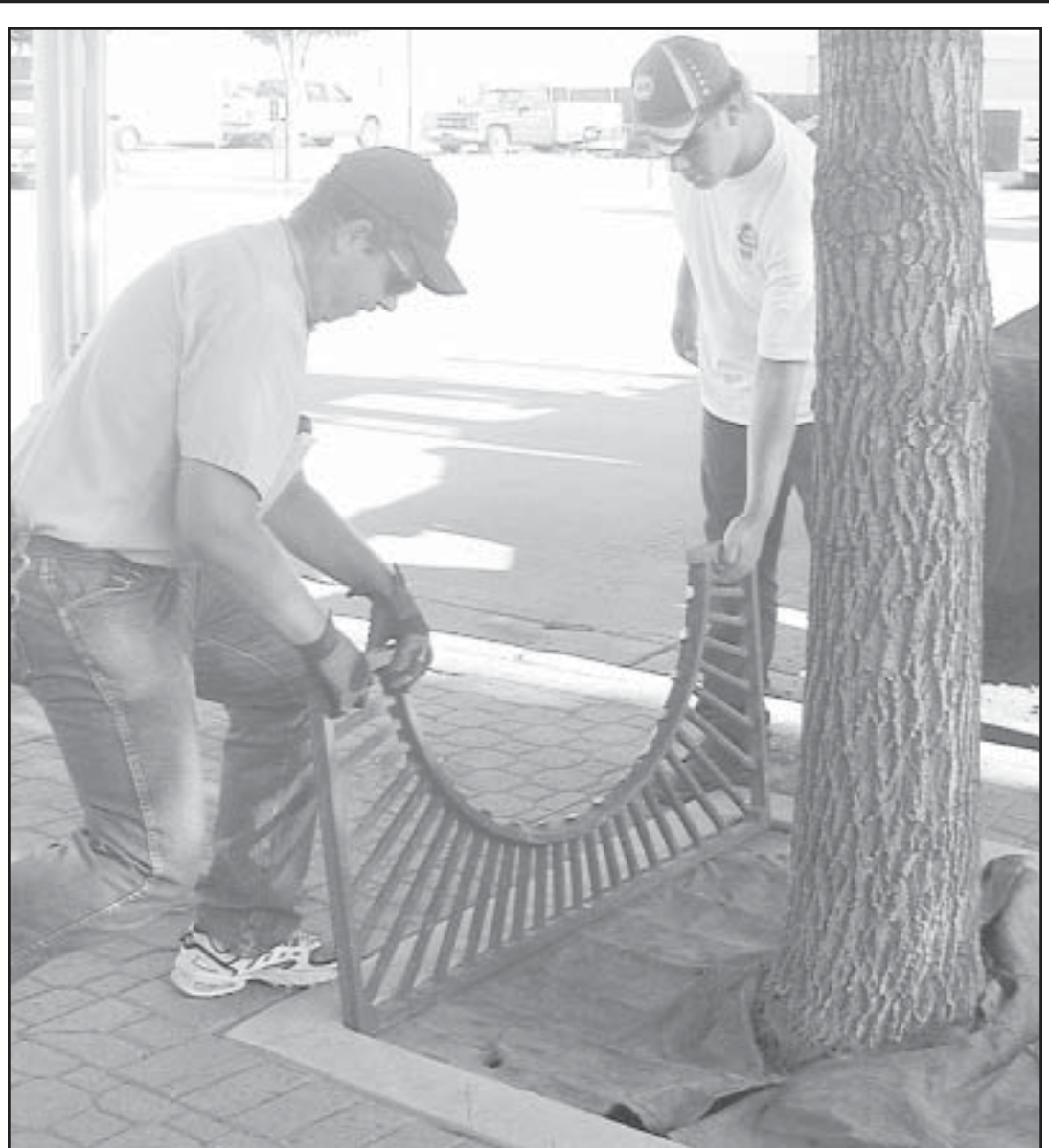
MAKING ROOM for the trunks of the trees on Main Street is keeping the city crew busy. Above, Mike Meyers and John Keller lay in the grate after making the cut.
