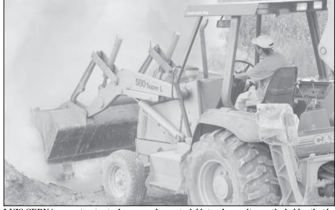
LUIS CERNA uses a tractor to dump surplus material into a burn pit near the bridge that he and his co-workers have completed north of Bird City. Herald staff photo by Casey McCormick
