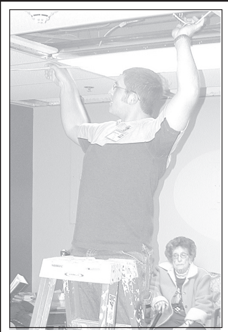
GOODLAND VO-TECH Electronics and Computer second-year students were at the Cheyenne County Hospital upgrading the computer wiring from a Category 3 to a Category 6. Pictured running wiring through the dropped ceiling is Gabe Gerber. Herald staff photo by Karen Krien
