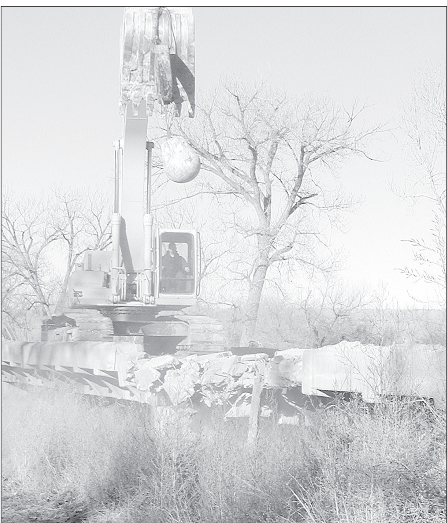
1935 BRIDGE IS DEMOLISHED — Greg Cahoj was operating the big crane which brought the 8-span, 8 foot bridge down Wednesday. The road was blocked but several people,
