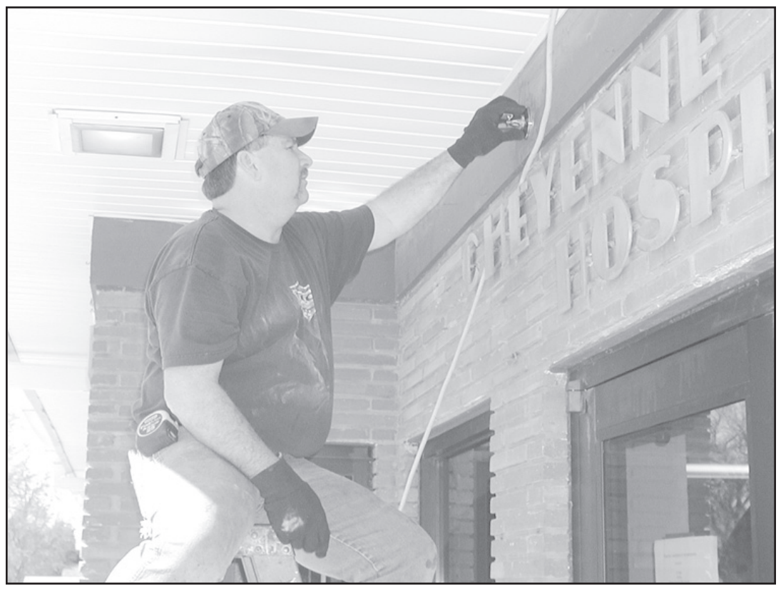
INSTALLING SPRINKLERS —Mac McCraw from American Fire, installs the new sprinkler system over the main entrance at the hospital. Herald staff photo by Casey McCormick
