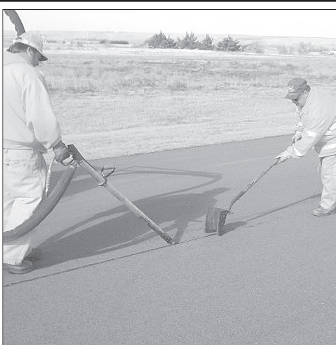
PATCHING THE CRACKS on the Cheyenne County runways. Bill Lee and Larry Zweygardt were among the state crew doing early maintenance to extend the life of the asphalt.
