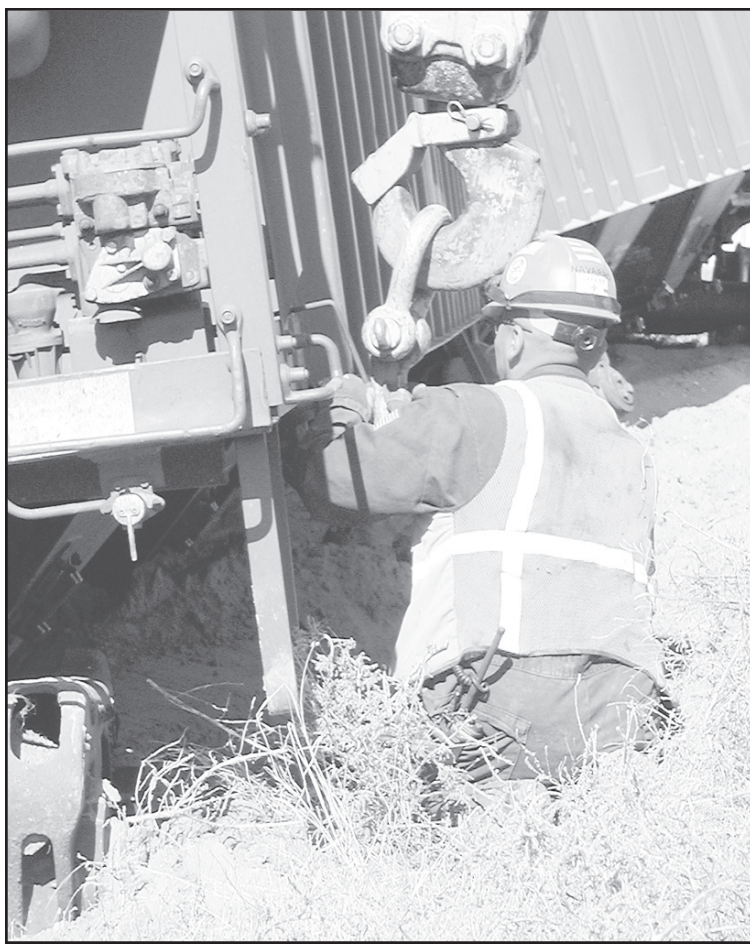
A PROFESSIONAL CREW arrived in St. Francis on Thursday and, within hours had the three cars back on the track. The foreman, at the top, directed the drivers in setting up the cars. Below, this worker makes sure the giant hook is attached.
