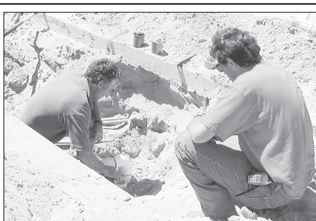
KELLY MORRIS and his helper were laying new pipeline at the Equity Station.
