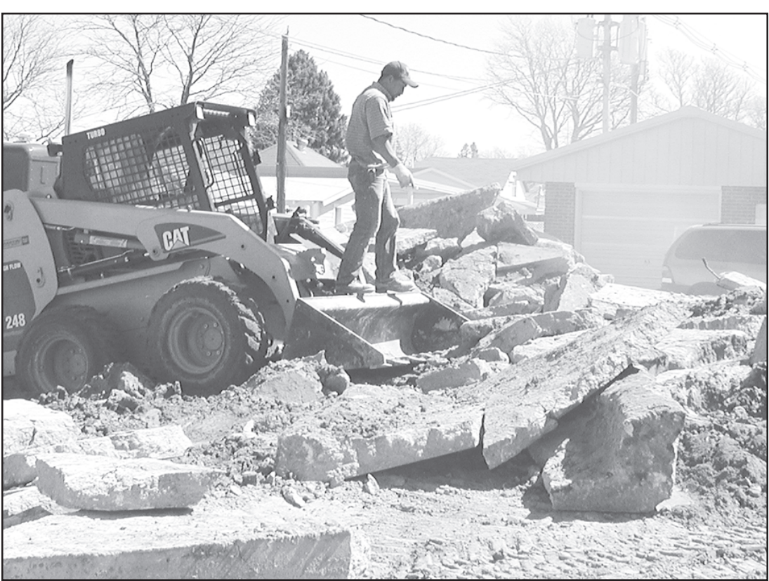
EMERGENCY ENTRANCE RAMP at the hospital is history. Workmen began tearing up the old ramp and a new ramp with ambulance garage will soon be seen. Herald staff photo by Karen Krien
