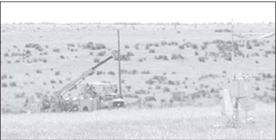
POLES SET — Prairie Lane Electric crew recently set the poles to bring in electricity for the automated weather observation system at the Cheyenne County Airport.
