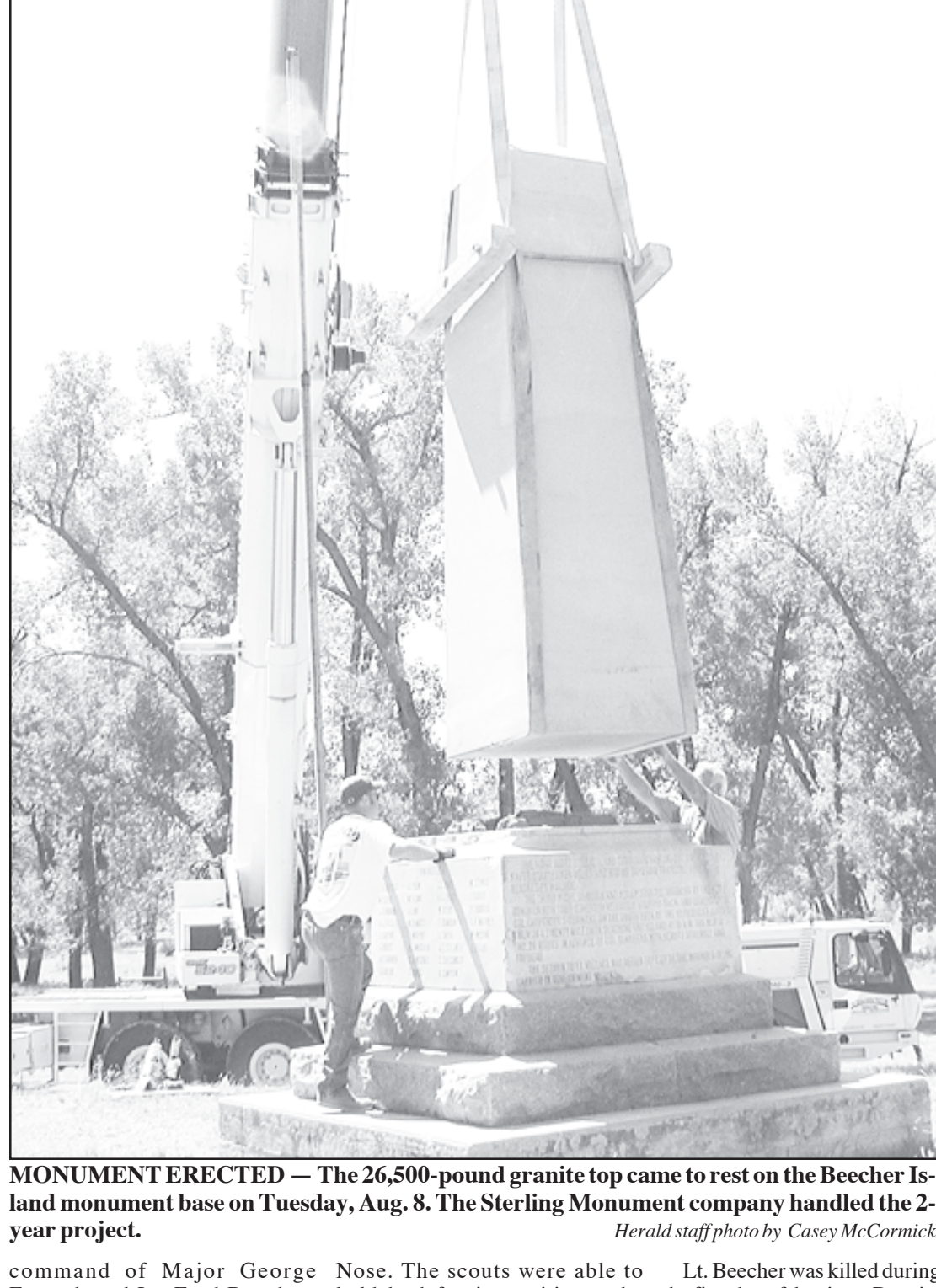
MONUMENT ERECTED — The 26,500-pound granite top came to rest on the Beecher Island monument base on Tuesday, Aug. 8. The Sterling Monument company handled the 2-year project.
