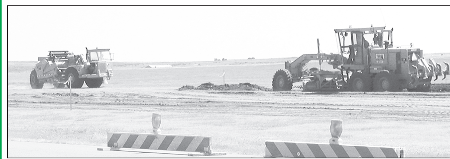
BIG EQUIPMENT is leveling the area in preparation for the apron (parking area) at the airport in St. Francis.
