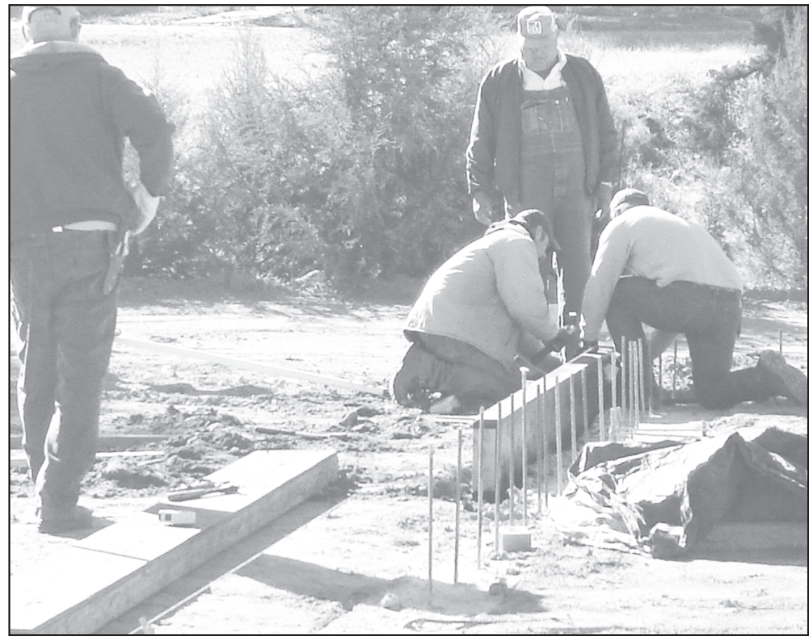
NEW EMERGENCY BUILDING has been started. Footings were poured on Monday. Ron Krien supervises some of the workers. Photo courtesy of J.R. Landenberger
