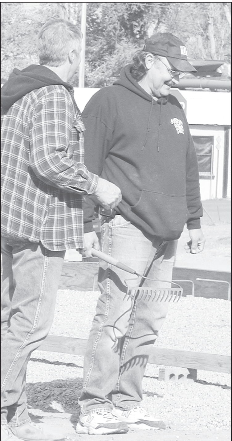
WORK IN PROGRESS — Dave Flemming and Scott Schultz are working on the emergency building site.
