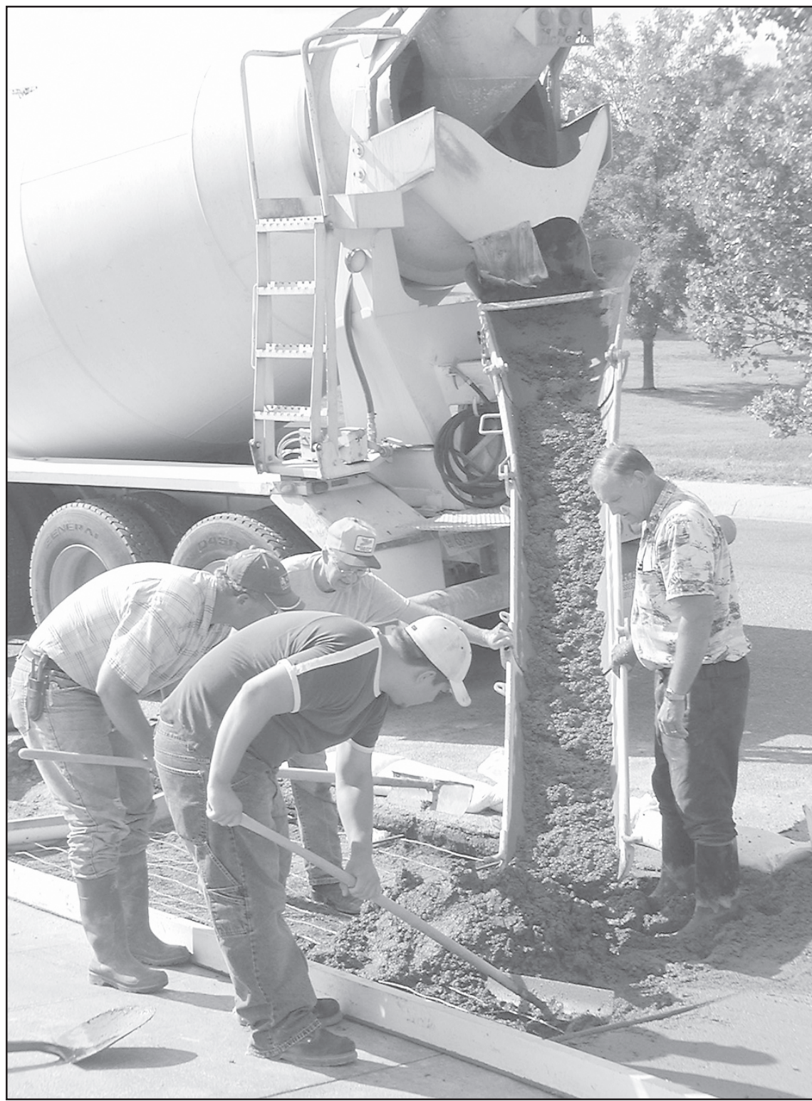
Members of the Colby Wesleyan Church poured concrete last week for the church's new, relocated parking lot driveway. The driveway work is the first of four phases of addition to the church.
