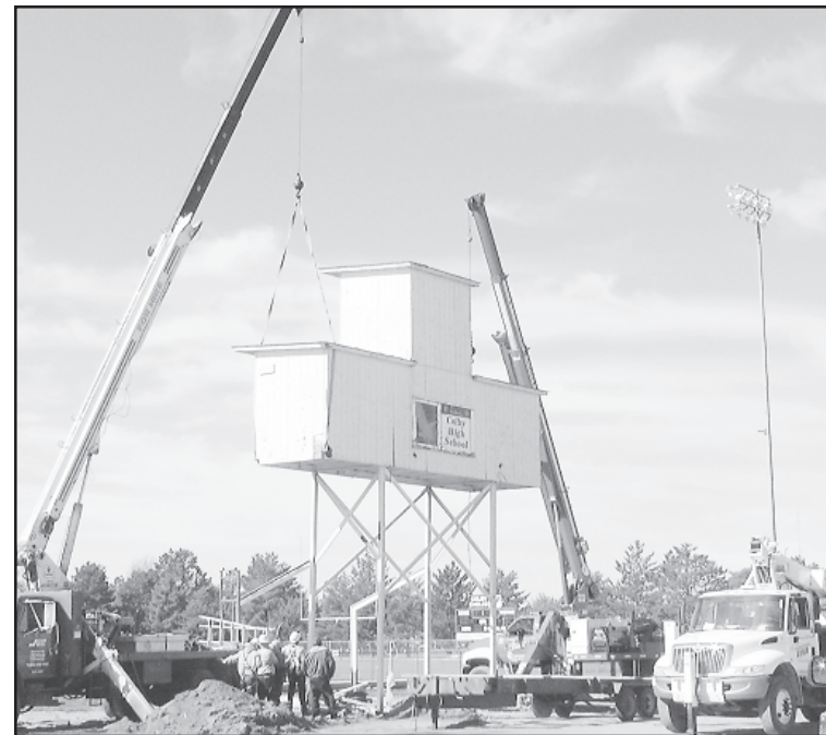
ABOVE LEFT: The old press box at Dennen Field was removed in April along with the old stands, to make way for a new stadium.
