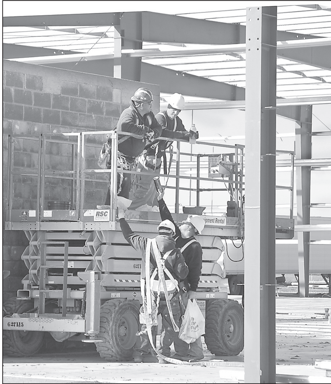
Before weather shut things down this week, a crew was working on the new home of Colby Implement, west of Truck Town and south of I-70.
