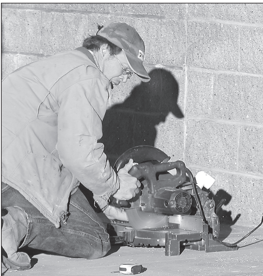
Work is moving along on the new Colby Implement building south of Interstate 70 on Horton Avenue. Tim Wilson of Colby Glass was installing the front doors this morning. The agricultural equipment dealership is hoping to move from its current location east of Colby around March 1.
