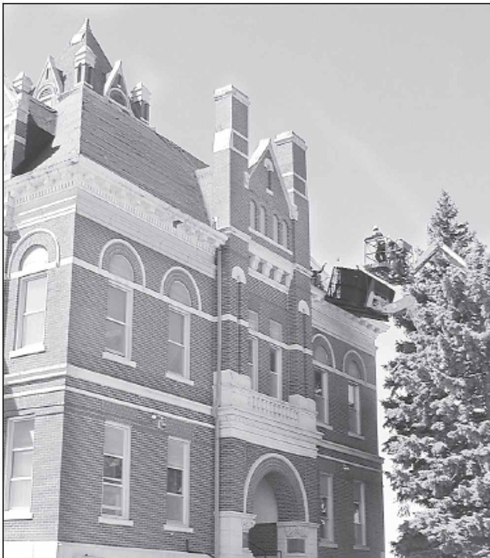
The hundred-year-old Thomas County Courthouse has undergone many repairs and renovations over the years, including these recent repairs to the building's roof.
