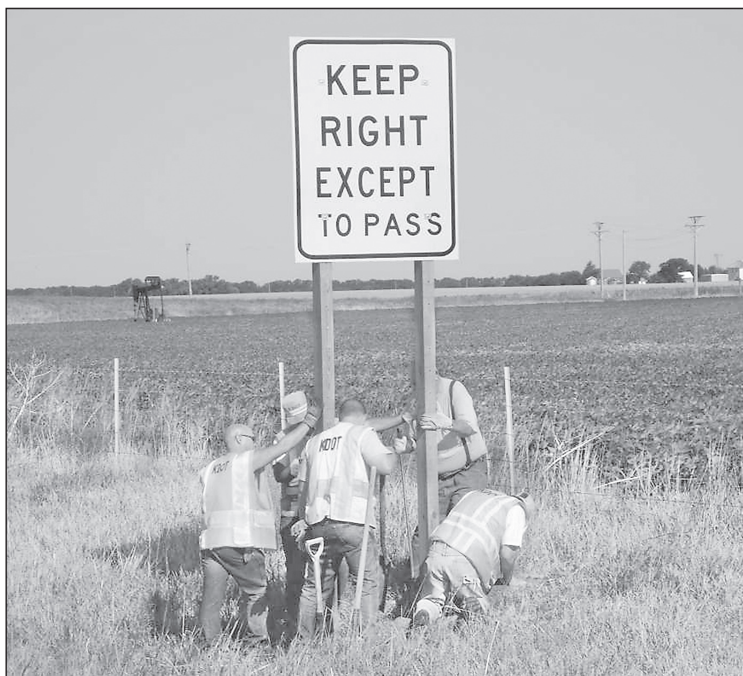
Crews from the Kansas Department of Transportation have installed nine new road signs in the last several weeks along the western portion of I-70. Two signs were installed in Thomas County, one at the Country Club Drive exit in Colby and one at the Levant exit. The signs remind drivers to keep in the right lane except to pass.
