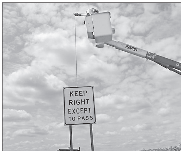
The locations for the new signs were chosen both for high traffic-volume and to space the signs out throughout the western stretch of I-70. No other signs are planned for northwest Kansas since I-70 is the only highway with more than one lane going either direction.
