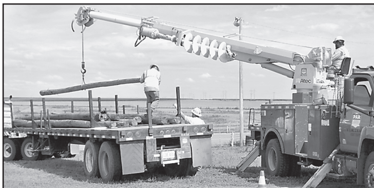
DEBBIE SCHWANKE/Colby Community College PAR Electric crew members unloaded donated poles at the Colby Community College horse arena.
