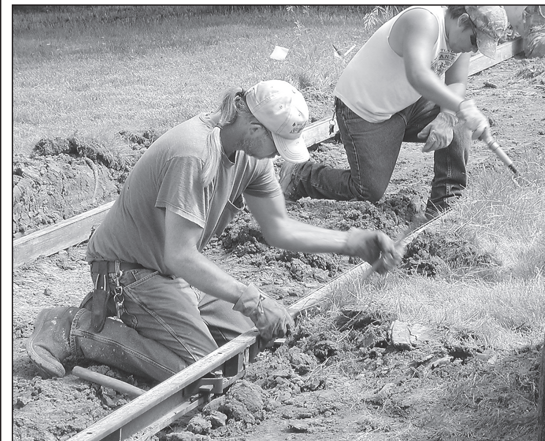
ANDY HEINTZ/Colby Free Press City workers Kyle Brogan and Steve Samuelson worked on extending the sidewalk on Range Avenue that will eventually run from Colby Community College to the stoplight at Range and Davis Avenue on Thursday.
