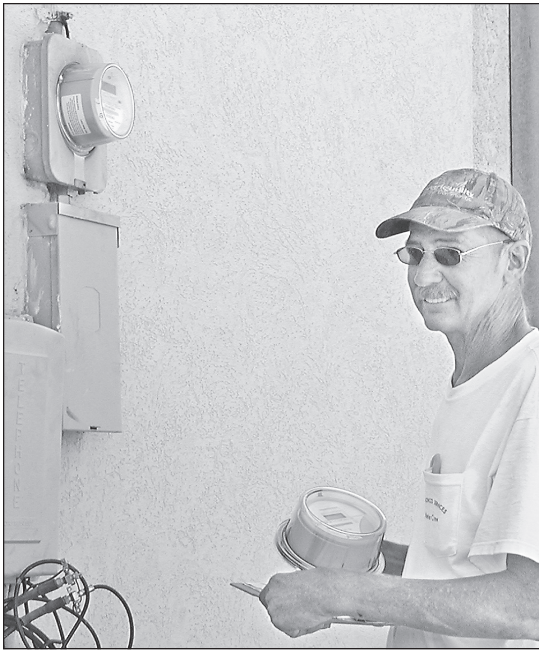
KATHRYN BALLARD/Colby Free Press Danny Braun of Florida switched out an old electric meter for a new one Thursday at Thomas County Insurance on Fifth Street. Braun works for U.S. Bronco Services, which subcontracted to install the meters for Johnson Controls Inc. and the City of Colby. The new meters are electronic and send information automatically, which means they no longer have to be manually read by city employees.
