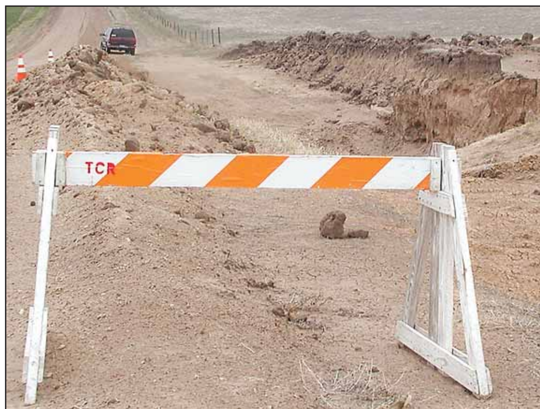
Sawhorse barricades and two cones are the only markers to warn drivers of a deep dug-out area on County Road 28 in North Randall Township.
