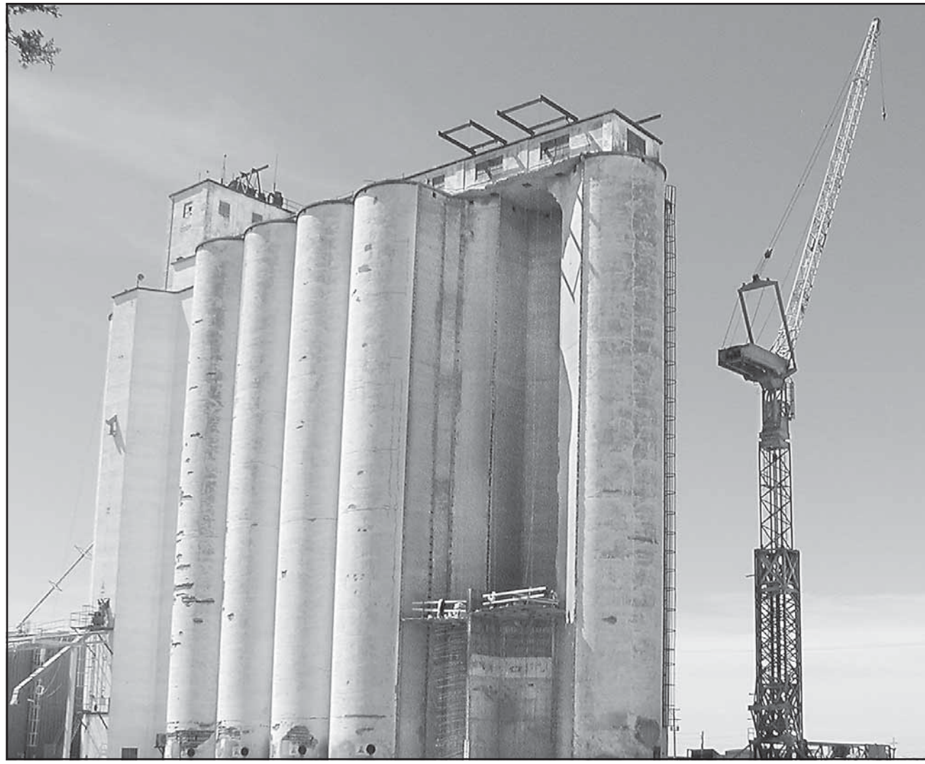
The Frontier Ag grain elevator in Oakley was showing signs of improvement Tuesday after it collapsed last November. SAM DIETER/Colby Free Press
