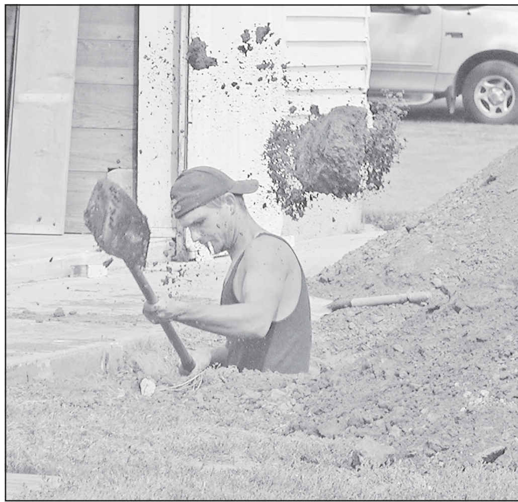
A worker helped dig out a pit Wednesday to connect the Cooper Barn to the city sewer system. The Prairie Museum of Art and History is working on a kitchen and rest rooms in the barn, located on the museum grounds.
